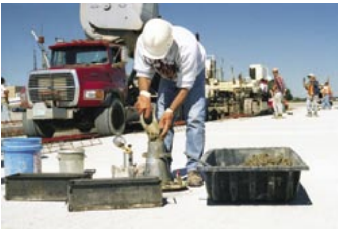
Individuals certified as Concrete Field Testing Technician—Grade I have demonstrated the knowledge and ability to perform and record the results of basic field tests on freshly mixed concrete, including slump flow testing (photo courtesy of the Ohio Ready Mixed Concrete Association)
